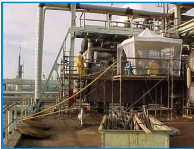
Operator Shelter with Reuse System
